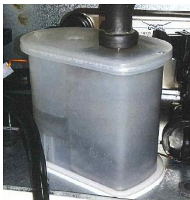
Dirty/blocked condensate trap
